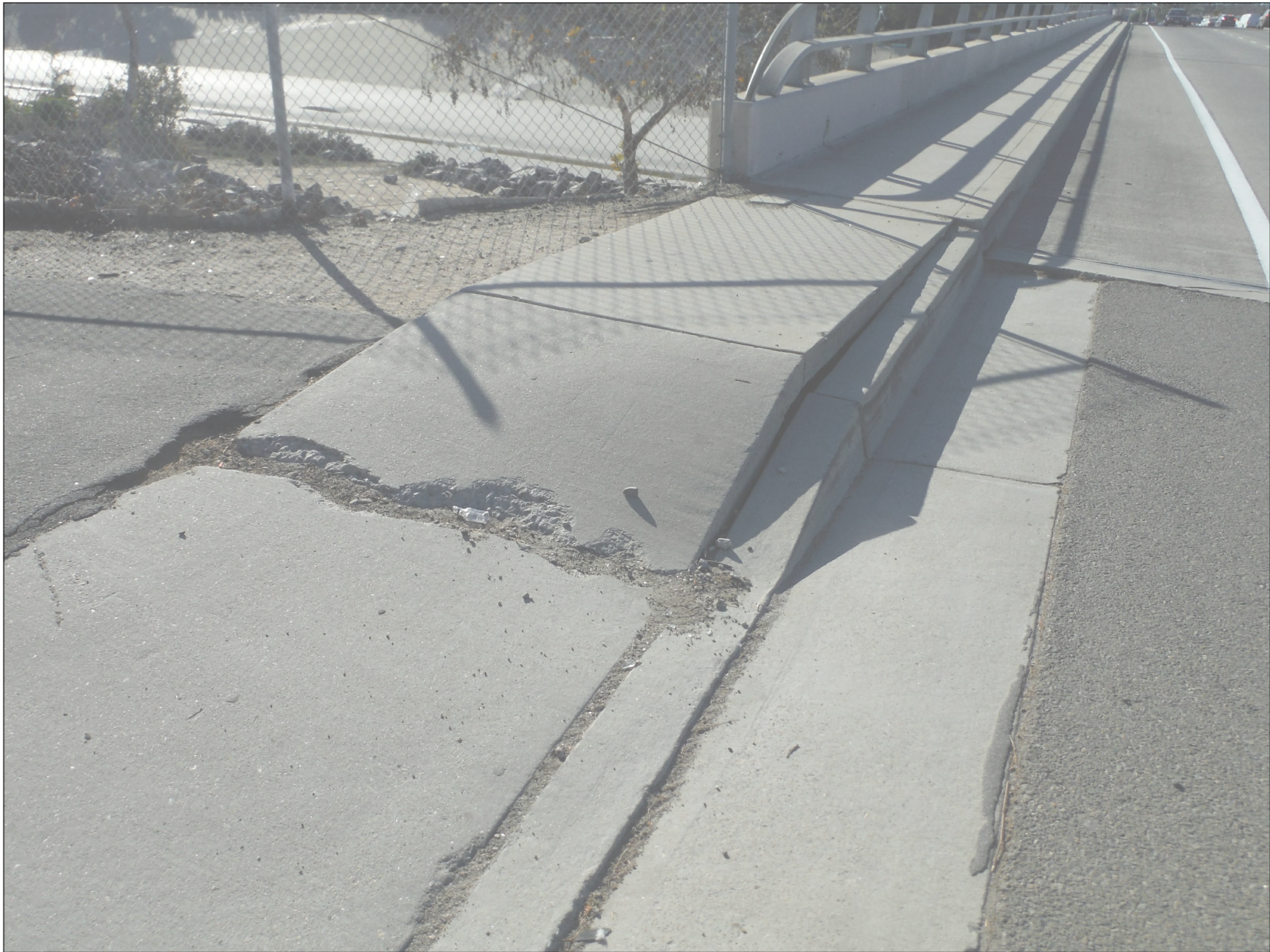
DAMAGED SIDEWALK SCALE: NONE
