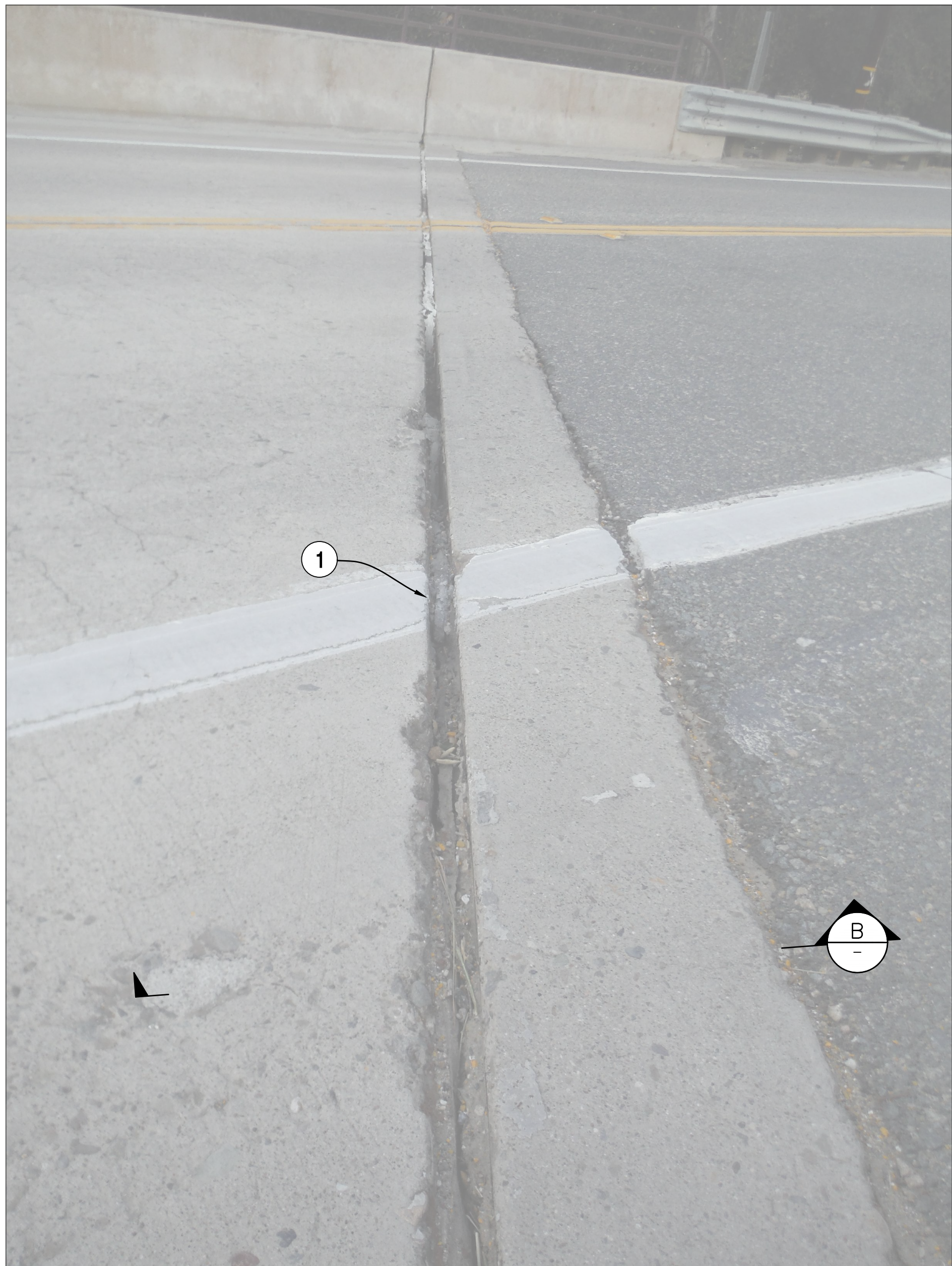
A C-001 VIEW OF DAMAGED JOINT SEAL SCALE: NONE
